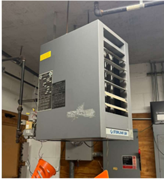
Existing furnaces and unit heater
