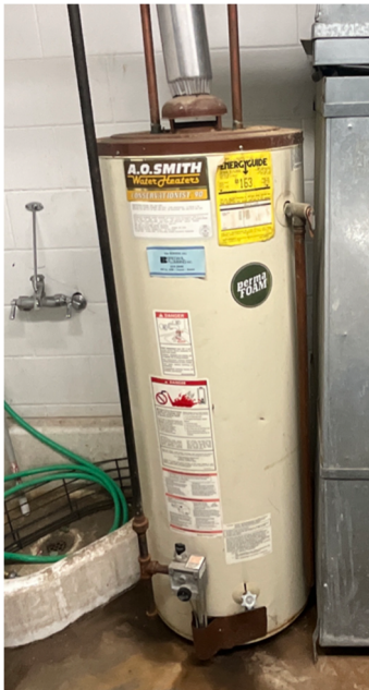
Existing Water Heater.
