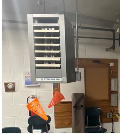
Existing Gas Unit Heater
