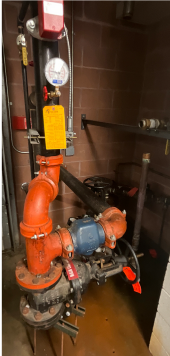
Main Water Service into Building
