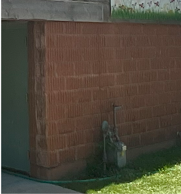
Existing Natural Gas Service.
